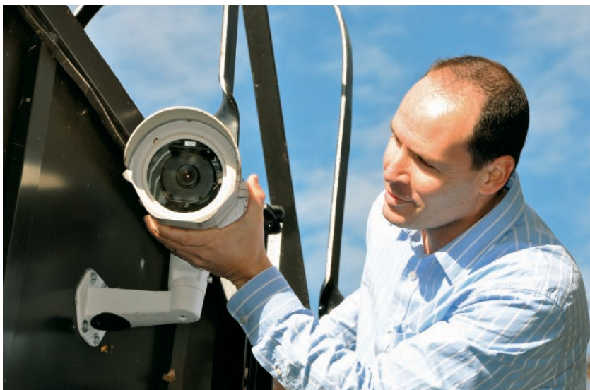
Idesco Senior Project Manager Simon Vizgan adjust the focus of one of the more than 25 Arecont megapixel cameras installed throughout SAR's campus and two main buildings. The solution helps ensure the welfare of the facility's approximately 1,300 students.
