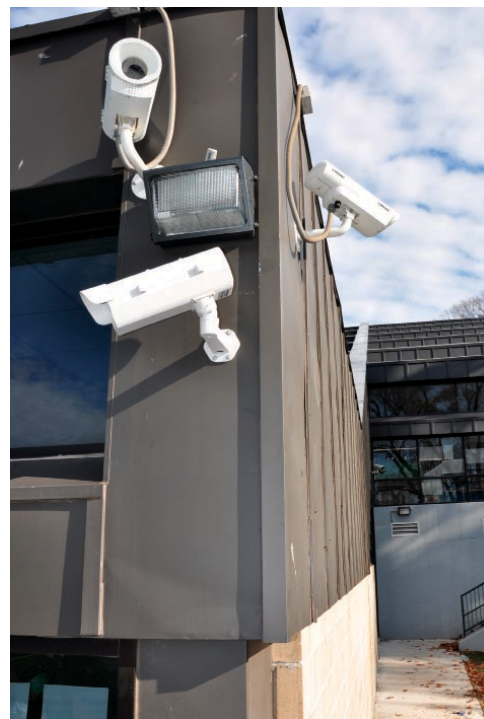
Five-megapixel cameras were situated to cover all angles, providing comprehensive surveillance for the school. Note conduit was still yet to be added to the cabling.
