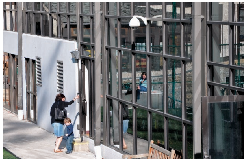
An Arecont's 180° megapixel dome camera mounted within view of one of SAR Academy's entryway/exits. The project included the installation of more than 25 new 1.3- to 5-megapixel cameras, which greatly enhance images when compared to the old analog system.
